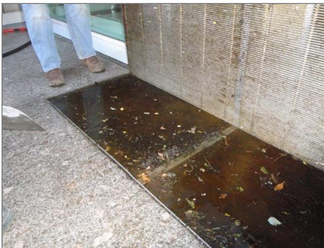
Figure 4 – Pan below grate at main entrance.
