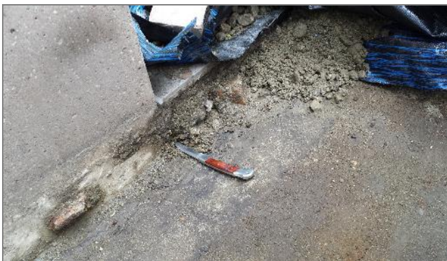
Figure 11 – Granit tile at main entrance is set on a low-strength concrete slab, which is sitting on a bed of rubble.
