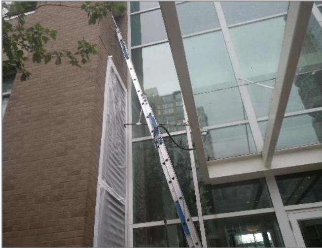
Figure 6 – Water penetration testing was performed at the brick to curtain wall interface immediately above leak location in lobby. The exhaust grate was covered in poly during test to confirm it was not the point of ingress.
