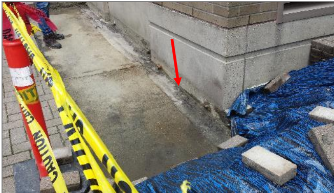
Figure 12 – Waterproof membrane extends under the pre-cast slab. The arrow indicates a location where there is water under the membrane.
