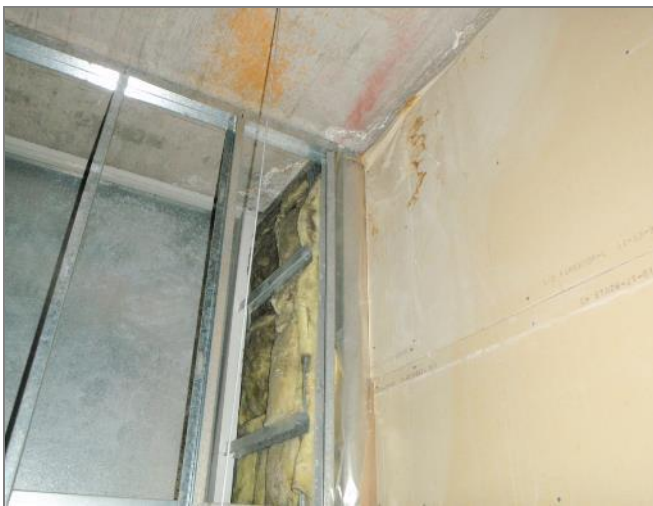
Figure 5 – Staining at brick to curtain wall interface above leakage location into lobby. This leakage path was confirmed through testing. Note, the staining was present before the testing was initiated.
