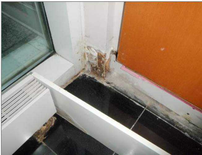
Figure 1 – Damaged gypsum sheathing and wood paneling at north side of lobby.
