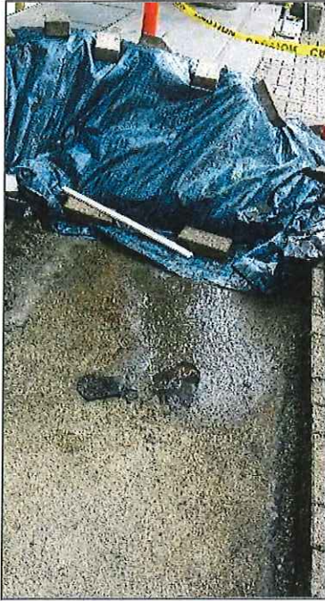
Figure 13 – Water under membrane on podium slab.
