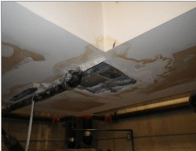
Figure 3 – Leakage into mechanical space below lobby.
