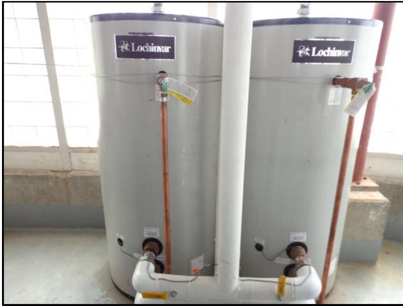
Photo No. 21: Domestic hot water storage tanks (typical)
