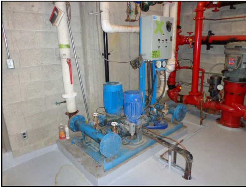
Photo No. 23: Booster pumps (typical) and fire pump
