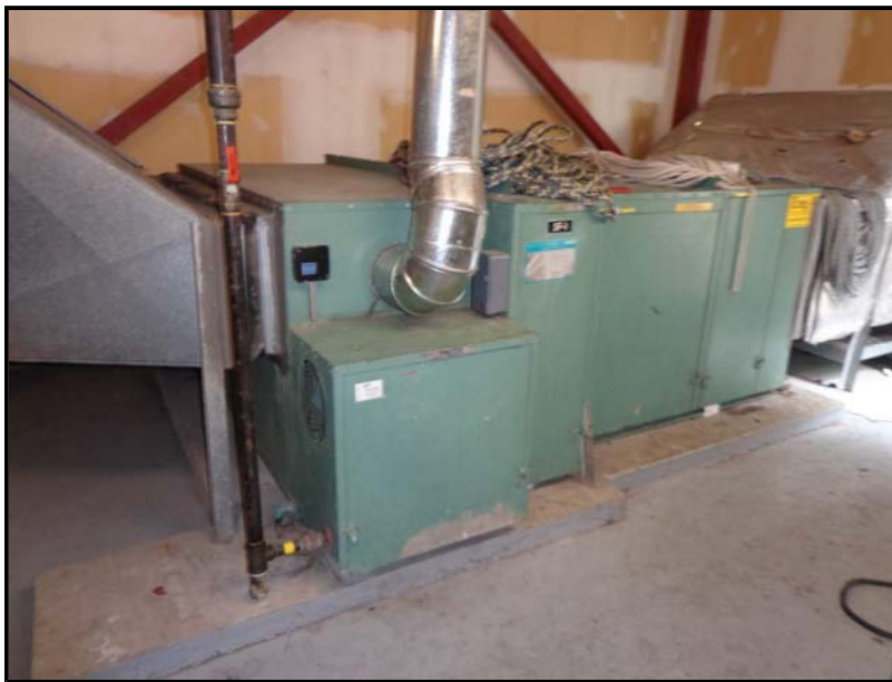
Photo No. 20: Make-up air unit (Beach Tower mechanical penthouse)
