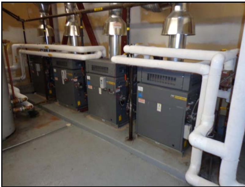
Photo No. 22: Boilers (Typical)
