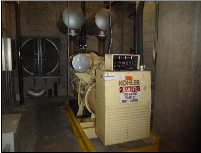
Photo No. 15: Emergency generator (P1 level generator room)
