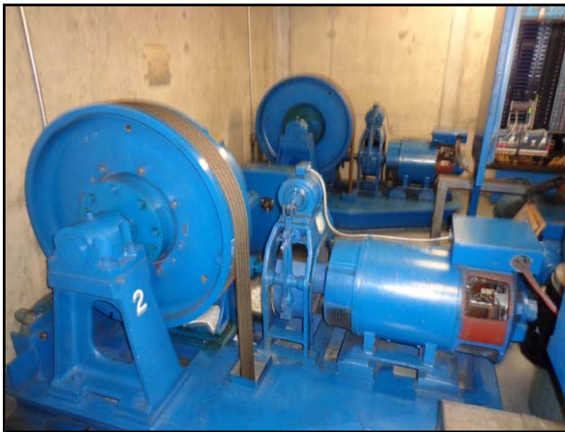
Photo No. 24: Elevator machines (typical)
