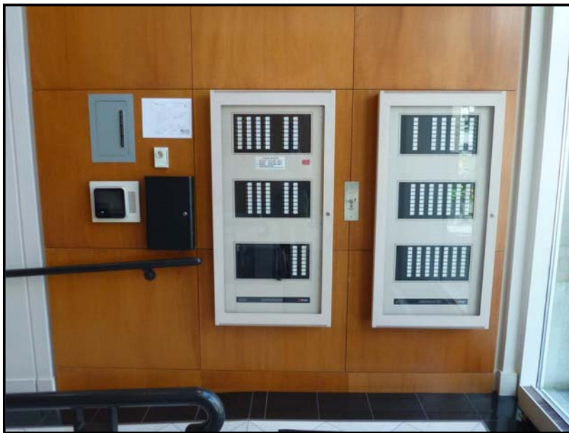
Photo No. 14: Fire alarm annunciator panel (Beach Tower lobby)
