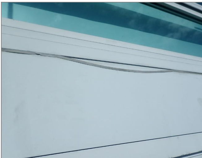
Figure 5.32 Sealant adhesive failure. Ocean Tower, Suite 1302, south elevation.
