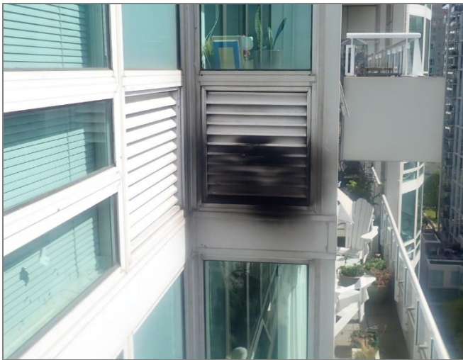
Figure 5.4 Stained fireplace vent. Beach Tower, Suite 1901, east elevation.
