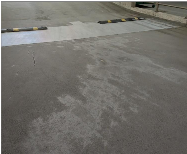
Figure 5.60 Existing wear at the traffic bearing membrane at the base of the east parkade entrance ramp.
