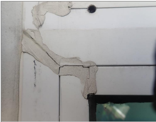
Figure 5.30 Cracked sealant at window mitre joint. Garden Tower, Suite 516, south elevation.
