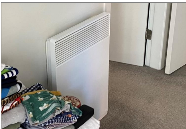
Figure 5.6 Electric wall convection heater at Townhouse 3.
