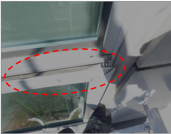
Figure 5.34 Misaligned window vent. Ocean Tower, Suite 1002, east elevation.
