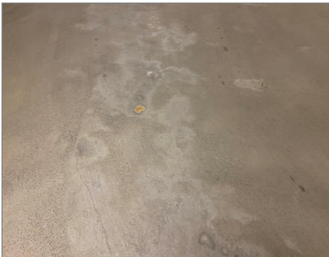
Figure 5.62 Localized exposed concrete substrate at the parkade traffic aisle. Parkade Level P2.
