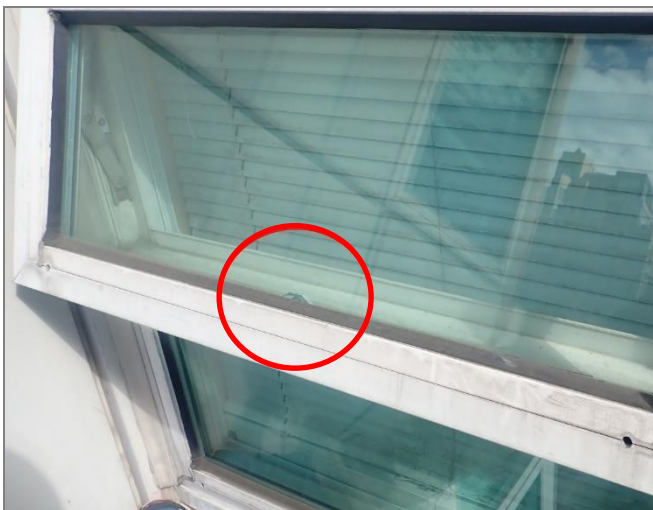
Figure 5.36 Damaged operable window handle. Ocean Tower, Suite 901, west elevation.
