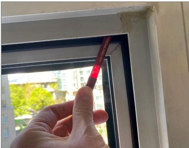
Figure 5.35 Misaligned awning window. Beach Tower, Suite 809, west elevation.
