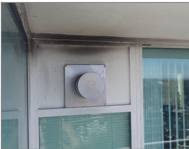
Figure 5.5 Stained fireplace vent. Ocean Tower, Suite 303, west elevation.
