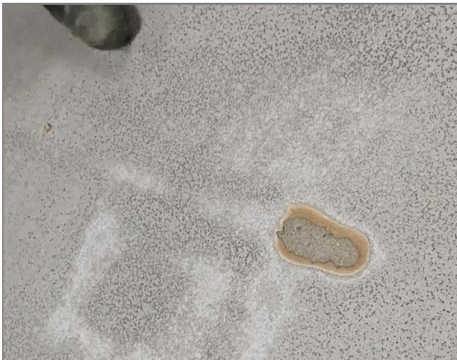
Figure 5.61 Localized exposed concrete substrate at the parkade traffic aisle. Parkade Level P1, Visitor Parking area.
